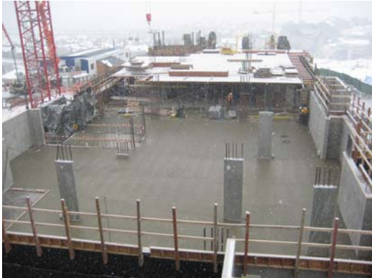
Construction workers for GE Johnson installed rebar at the new Edgemont condominium project during a frigid Christmas Eve morning Wednesday. The Sheraton Steamboat Resort and Steamboat Grand Resort Hotel are visible in the background. — Photo by Tom Ross
